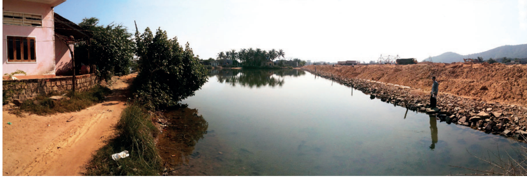
Photo 14. View of the new residential area (right) under construction near barrage No. 1.
