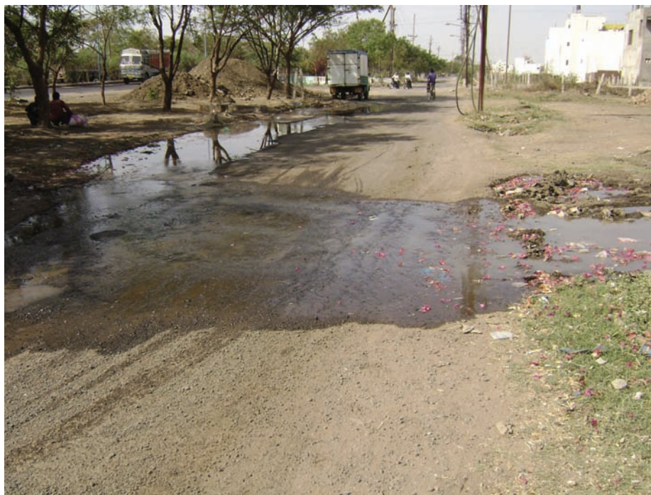
Drinking water pipeline leakage. © ISET
